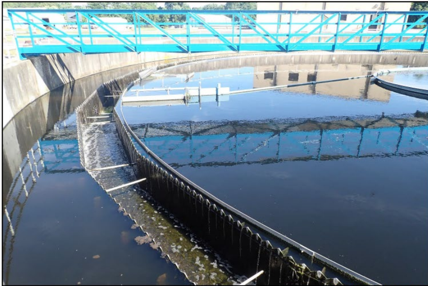
Lancaster Water Pollution Control Facility
