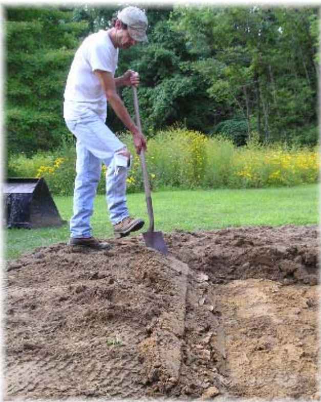
You can dig your rain garden by hand or use a backhoe. If you use a backhoe to dig your garden, avoid driving it on the garden site to minimize soil compaction.
