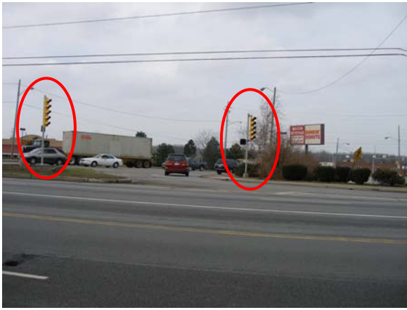
The pole-mounted traffic signal heads are intended to control traffic in the channelized right turn lane on the US20 westbound approach. They, however, operate in tandem with the signals mounted on the mast, which causes some confusion to drivers.
