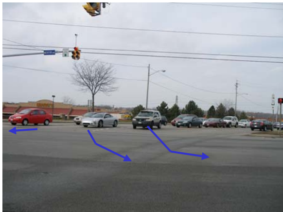
Absent are lane guide markings within the intersection to guide the double left turning movements from the SR306 southbound approach to US20 eastbound
