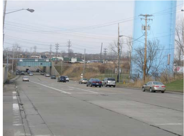
Faded/worn out lane and stop bar markings
