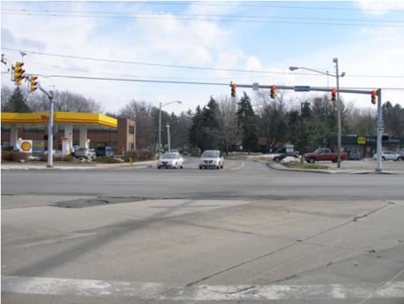
Faded/worn out lane and stop bar markings
