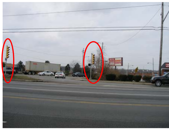
The pole-mounted traffic signal heads on the pole to the left, within the island, is intended to control traffic in the channelized lane as evidenced by its placement and location far to the right of the edge of the roadway for through traffic.
