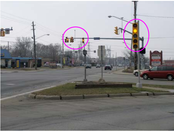
The pole-mounted signals, intended for the channelized right-turn lane, and the mast-mounted signals, intended for the through and left-turn lanes, operate in tandem causing the production of conflicting signal indications, shown in the photos below.
