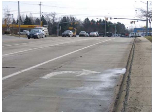
Faded/worn out lane markings and lane assignment arrows
