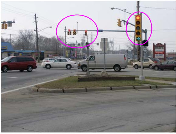
The pole-mounted signals, intended for the channelized right-turn lane, and the mast-mounted signals, intended for the through and left-turn lanes, operate in tandem causing the production of conflicting signal indications as shown in the photo. The signal heads mounted on the pole on the right of the road across the one shown in the photo display the same indications, hence the confusion.
