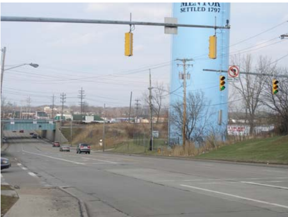
Faded/worn out lane, stop bar, and cross walk markings
