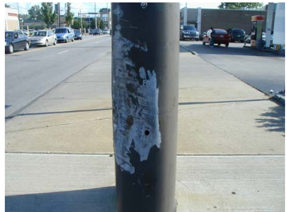
Damage to poles due to collision with turning vehicles
