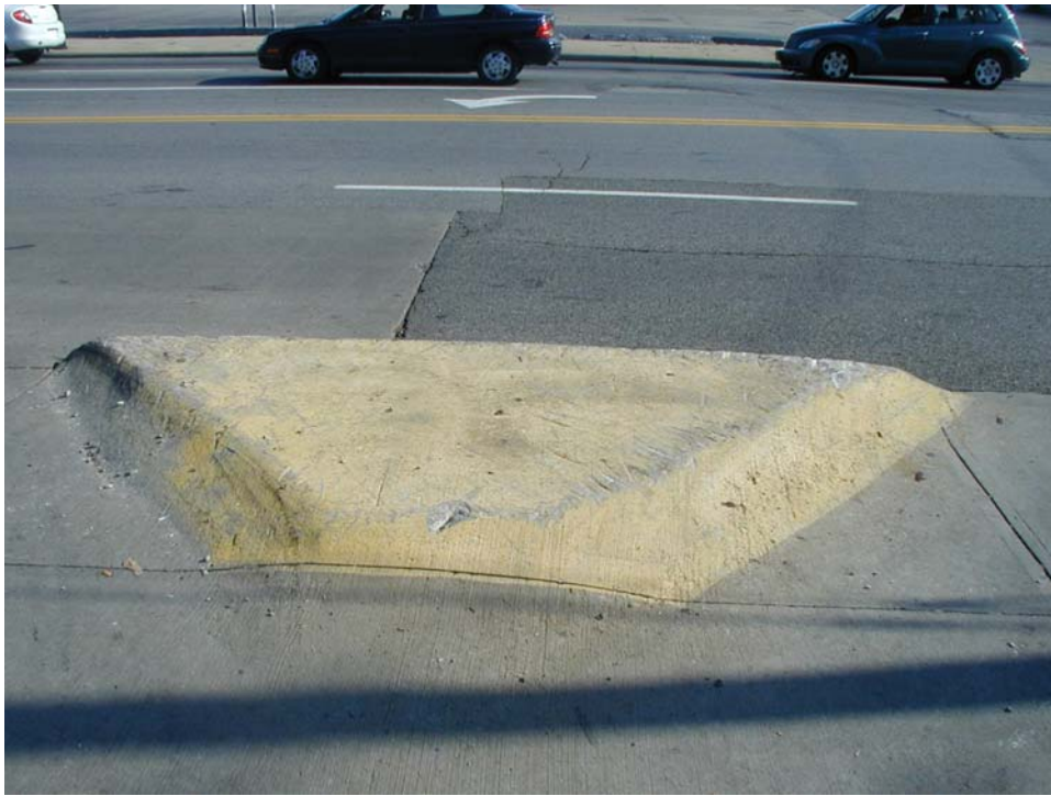
Raised island within the driveway of the BP gas station fronting Harvard Avenue to regulate right-in/right-out traffic movements
