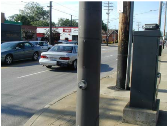
Missing pedestrian crossing actuation button and crossing orientation signs
