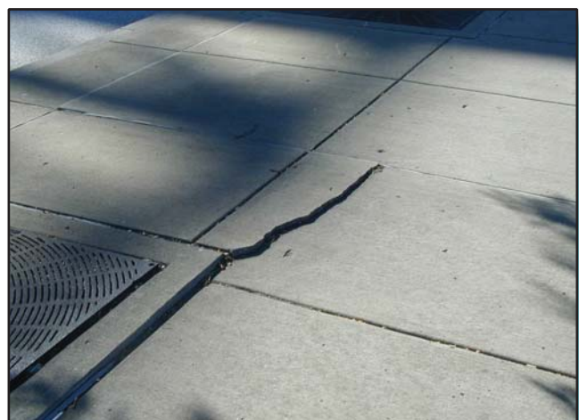
Picture 18: Damaged sidewalk
